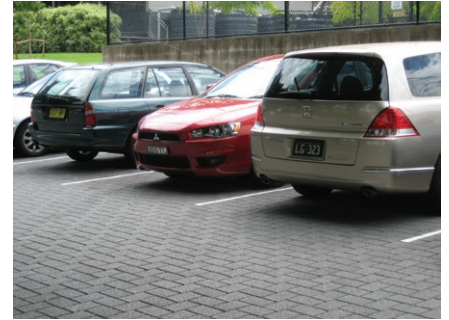
Permeable paving in carpark reduces and filters surface stormwater run off (Photograph: HydroCon Australasia hydroston.com.au)
